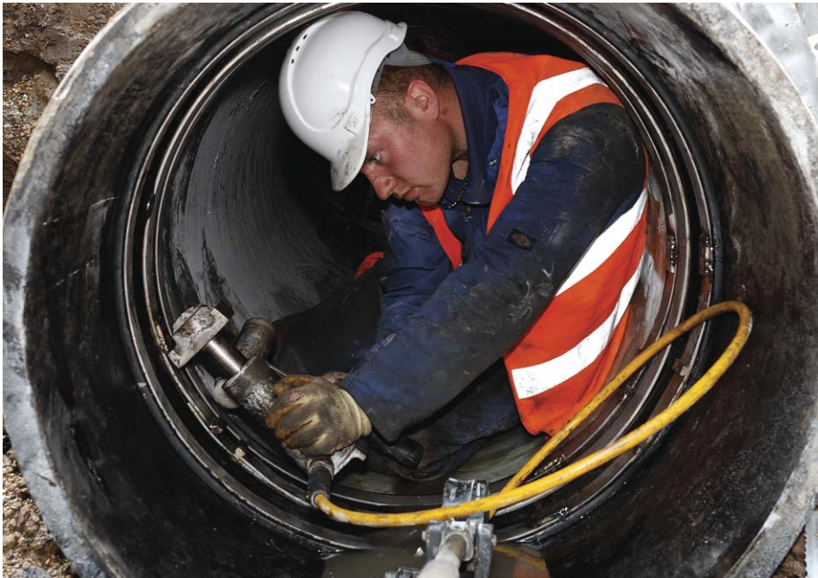
A PressureCIPP liner being installed into a 800mm diameter pumping main sewer at Wisbech in Cambridgeshire
