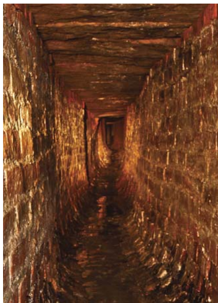
The failing U shaped sewer prior to lining
