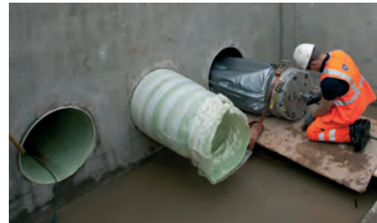
EcoCIPP liners in place in each pipe. One finished, one awaiting trimming and the third being prepared for inflation
