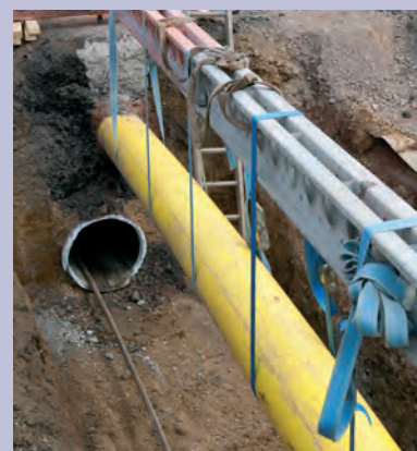
One of the access pits, showing the proximity of other services to the pumping main.
