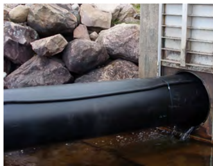
The new pipe is pushed into the host pipe. One of the three grouting tubes can be seen on the top of the new pipe.
