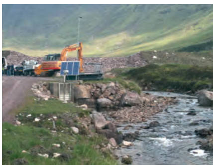
Looking up Russel Burn towards the new dam. The raised penstock of the outlet pipe is to the right of the track.
