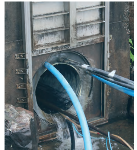
The newly installed pipe showing the grouting tubes, pushing rod and air line for the patch liner
