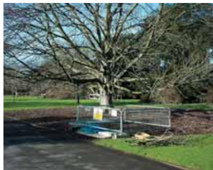
This 200 year old Indian Chestnut was left undisturbed as a 45m pipe burst was installed from the manhole.
