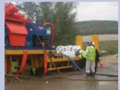
Perco mud mixing and recycling plant
